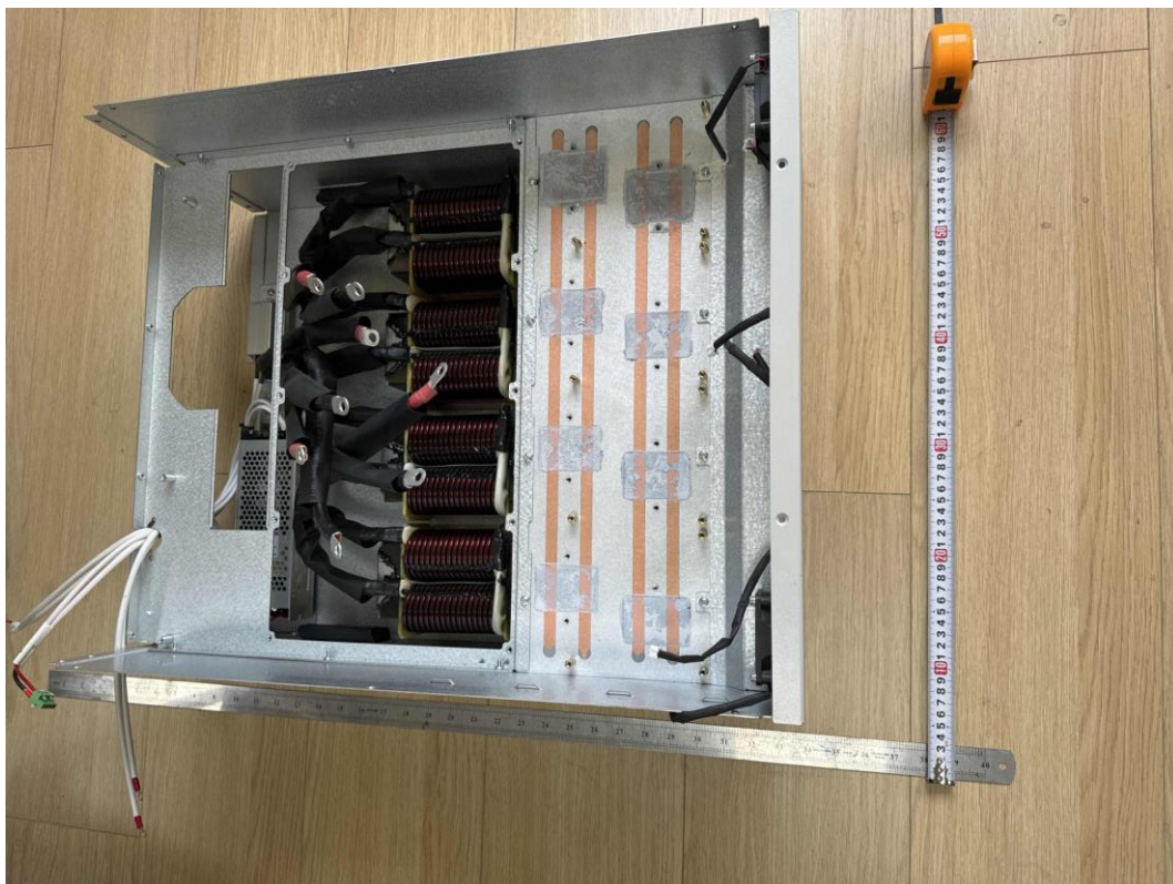
Figure 12 Inside view of enclosure without PCBs
