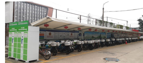
Street charging station
