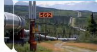
Pipeline for NICO
