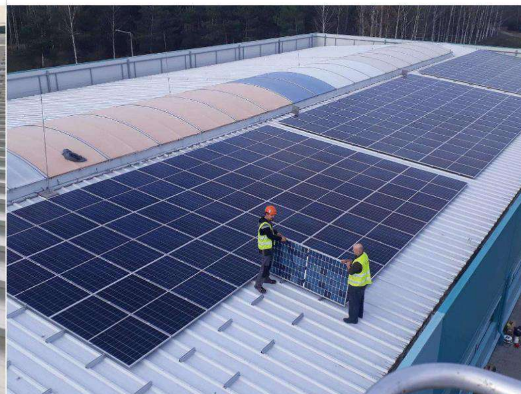
Metal Roof Mount-Poland
