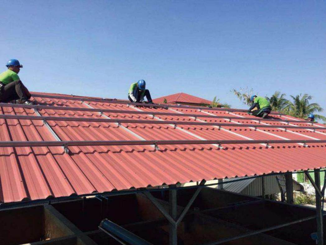
Metal Roof Mount-Cambodia
