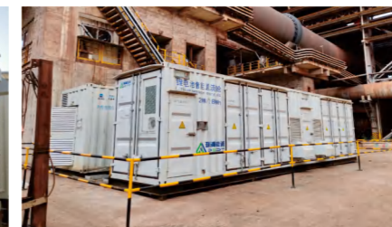
莫罗瓦利(IMIP)园区118MWh A project of 118 MWh in Morowali Park, Indonesia
