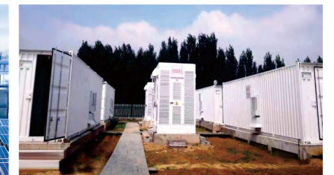
山东新泰10MWh光伏储能项目 A solar energy storage project of 10 MWh in Xintai, Shandong
