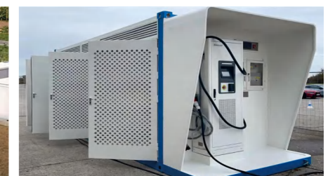
德国、法国、西班牙光伏储能项目 Solar energy storage projects in Germany, France, and Spain
