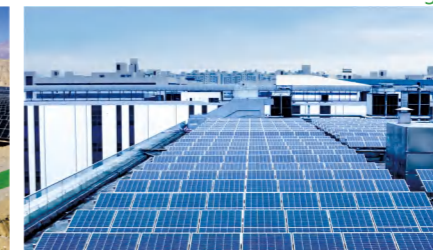
温州 3 MWh光伏储能项目 A solar energy storage project of 3 MWh in Wenzhou, Zhejiang
