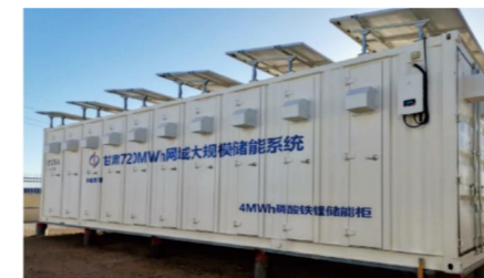
A Solar Energy Storage Project of 12 Mwh In Guazhou, Gansu
