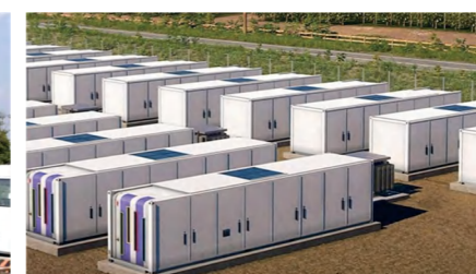
A Solar Energy Storage Project of 200 Mwh In Texas, U.s.
