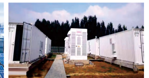
A Solar Energy Storage Project of 10 Mwh In Xintai, Shandong
