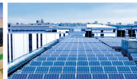
A Solar Energy Storage Project of 3 Mwh In Wenzhou, Zhejiang
