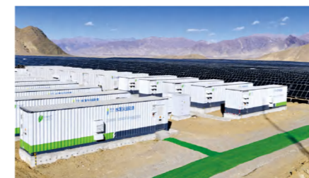
A Solar Energy Storage Project of 5 Mwh In Sangzhuzi District, Shigatse, Tibet.
