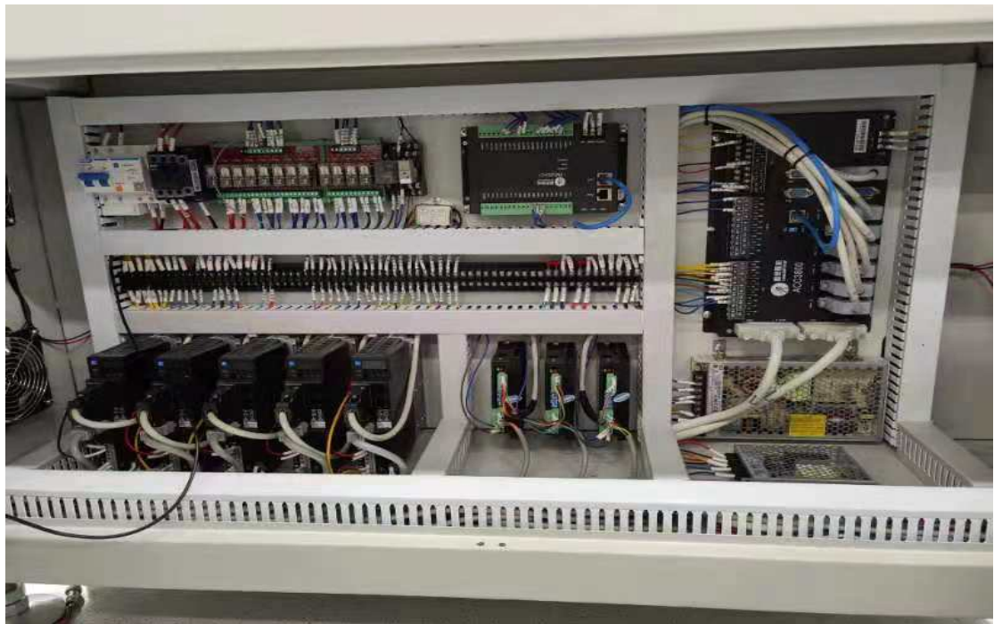
Figure 10- 7 Control the electric box
