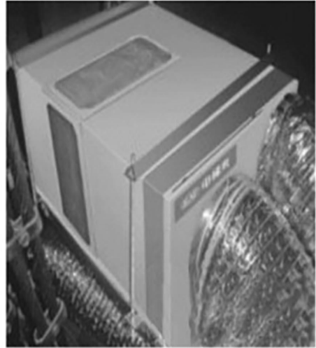
产品安装完工 Air conditioner installed successfully
