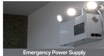
Emergency Power Supply
