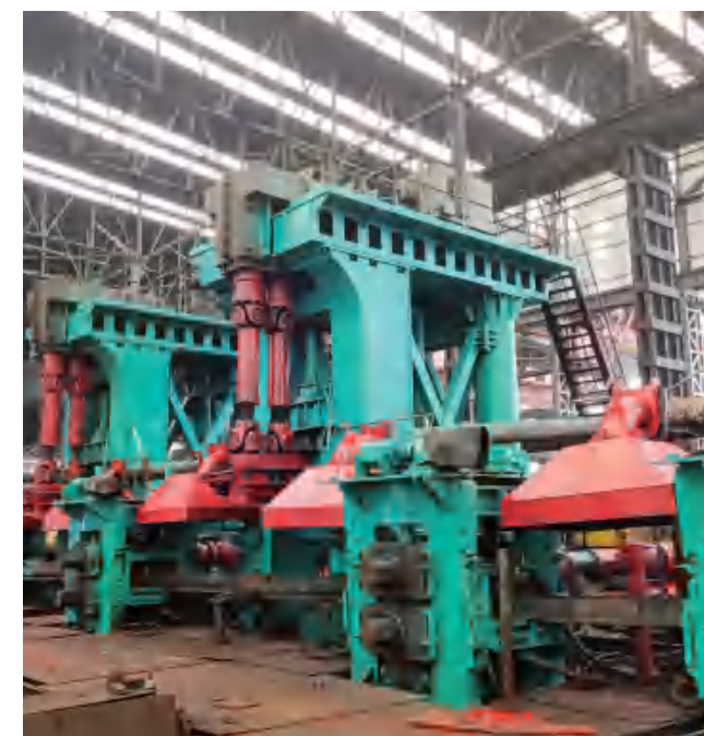
Hot rolling production line
