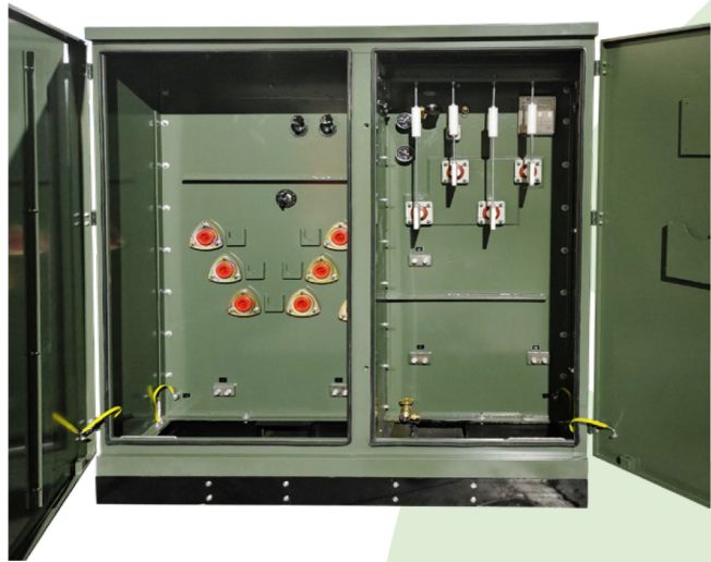
▲ Loop Feed Pad Mounted Transformer
