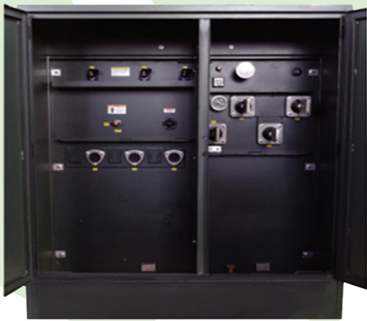
▲ Radial Feed Pad Mounted Transformer
