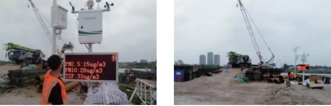
Air Quality Grid Monitoring
