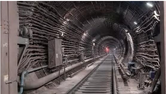
Underground Pipe Corridor
