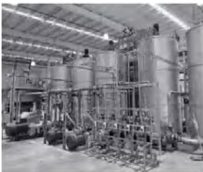
大型纸塑制浆系统—湿压示范线 Large Pulping Systems
