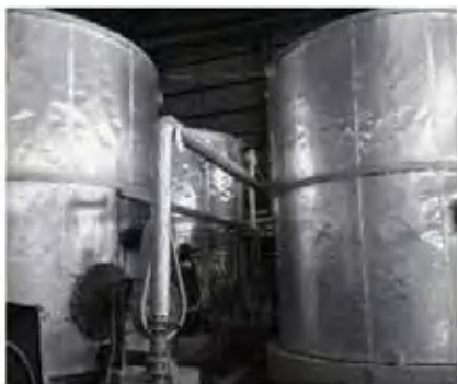
小型纸塑制浆系统—干湿压示范线 Small Pulping Systems
