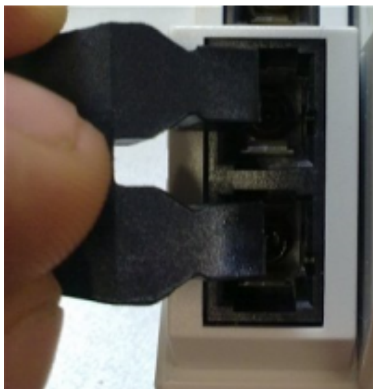
Figure: Blind plugs in unused sockets
