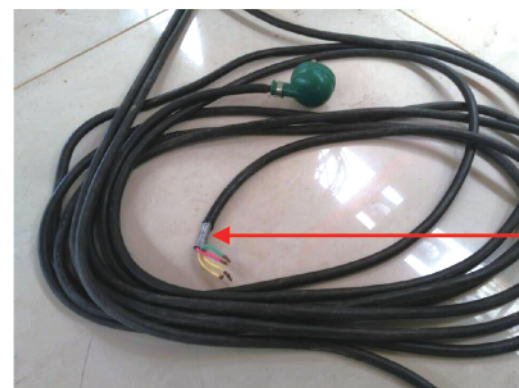
The power cable
