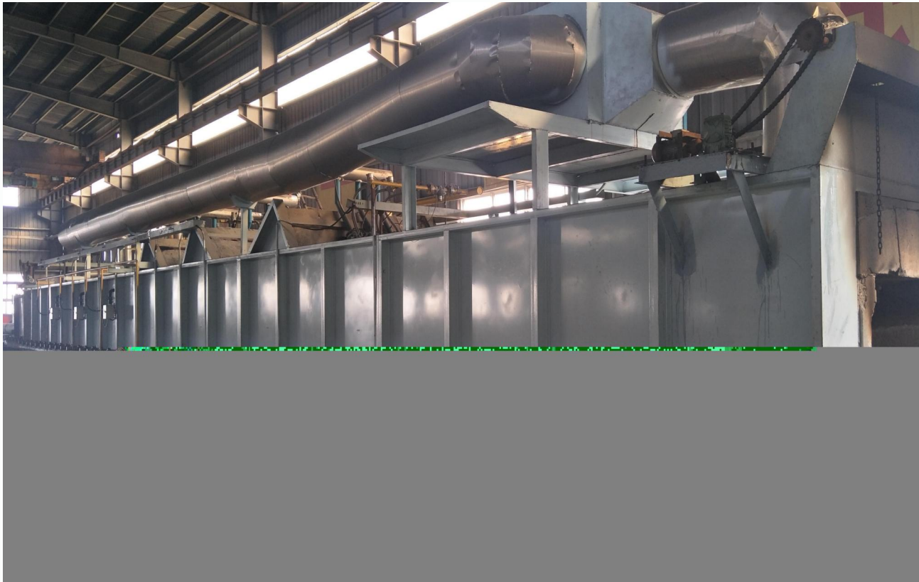
Natural gas annealing furnace (Automatic temperature control)
