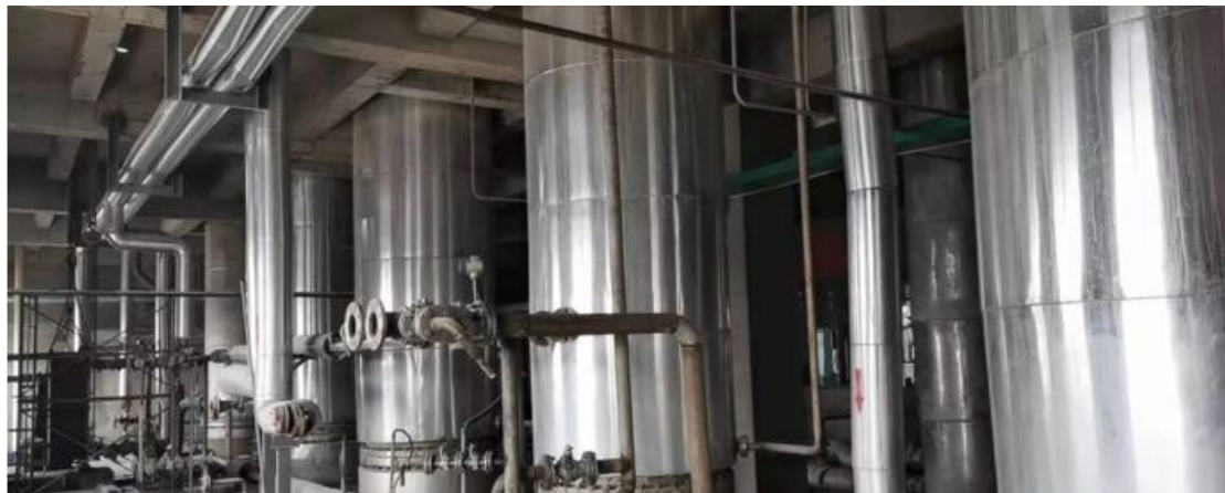
Potassium nitrate production line of 170,000 tons / year using ion exchange process (high standard molten salt material) )
